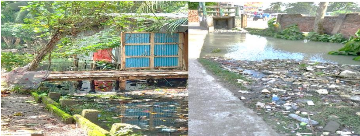
Figure 3: Conditions of drainage system: encroachment (left) and garbage dumping (right) (source: Field visit in December 2019)
