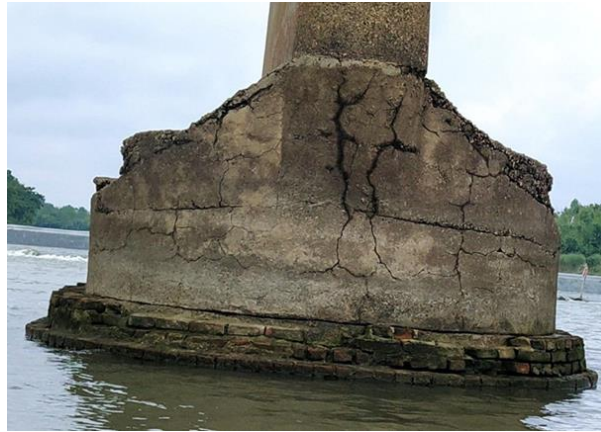
Figure 3: Damage in pier of Mohonpur Bridge
