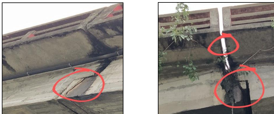
Figure 4: Damage in Drop-in-girder part of Mohonpur Bridge
