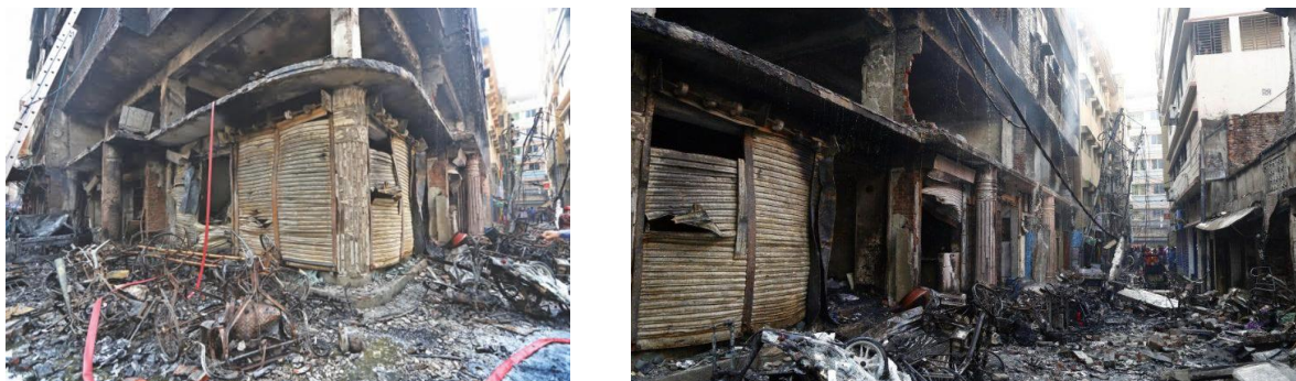
Figure 2: Concrete structures after Nimtoli fire incident ( in 2010, source-online news portal )
