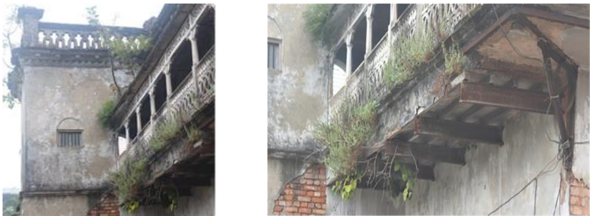
Figure 3: Biological colonization (Top), Timber supports on roofing (bottom) (Captured by Author, October 2021)
