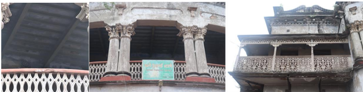
Figure 2: Kori-borga roof (left-side), Structural features of Agrani Transport Limited (Captured by Author. October 2021)
