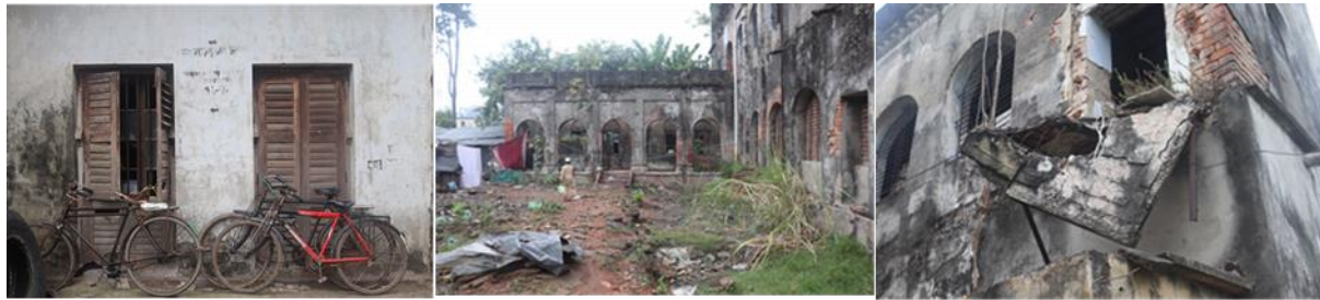
Figure 6: wooden windows details (left), backyard condition views (right) (Captured by Author, October 2021)
