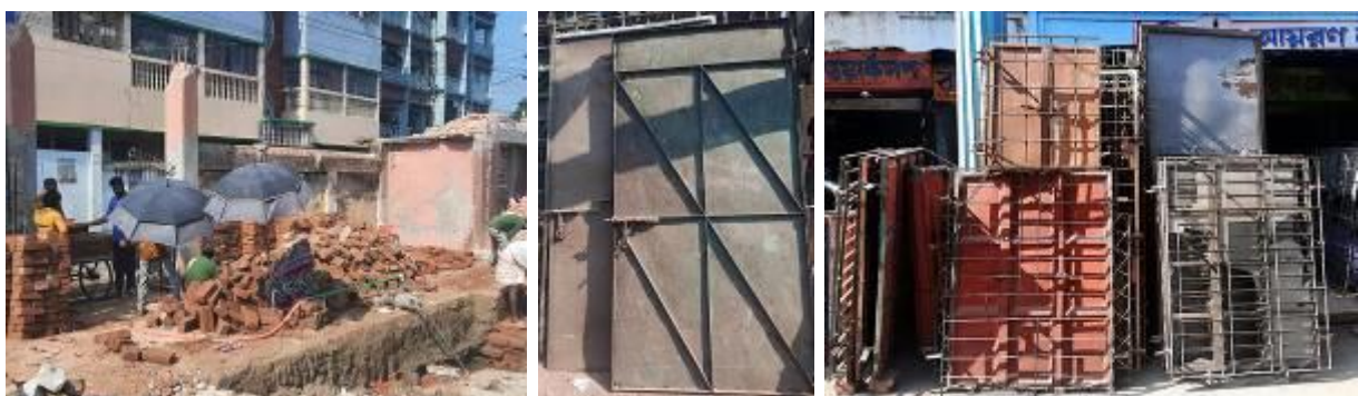
Figure 3: Worker remove plaster from the brick (Left), the old gate and grills are displaying in front of the shop for selling (Captured by Author, October, 2021)
