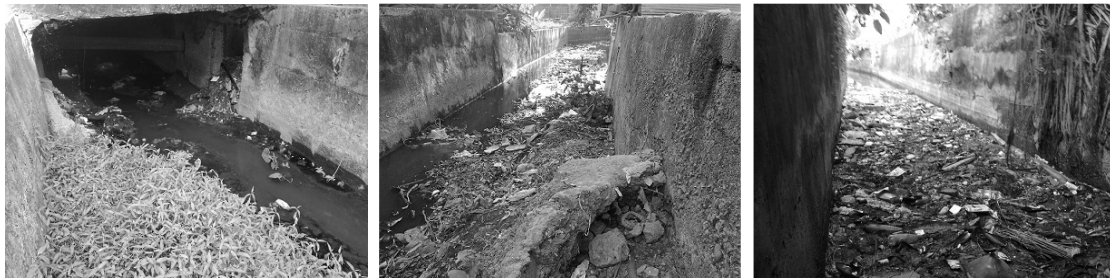
Fig 2: Condition of some outlets over Mayur river
