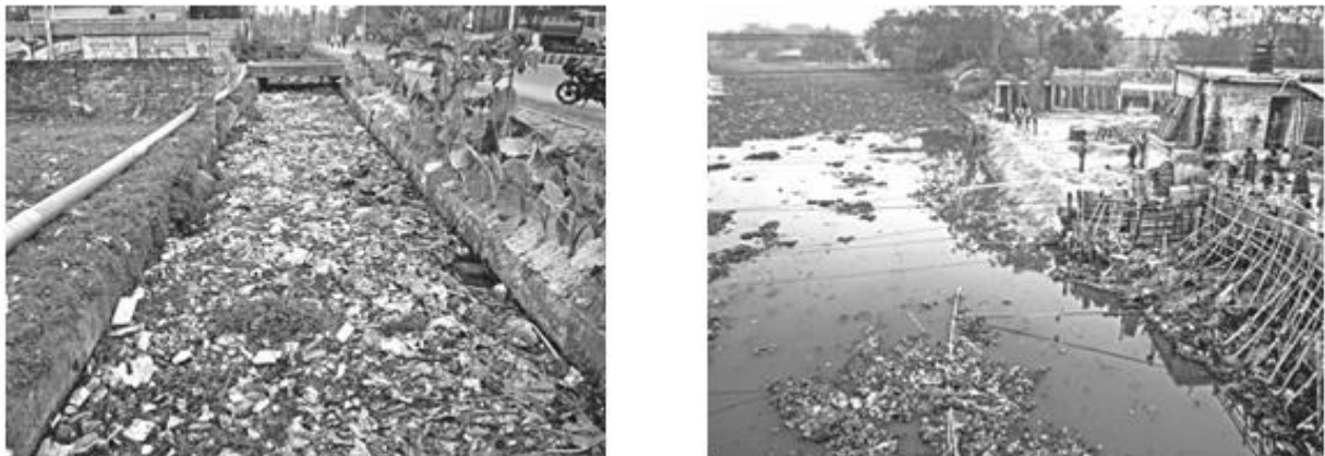
Figure 2: Conditions of drainage system: garbage dumping (left) and blockage of natural drainage (right). (Source: Field visit)
