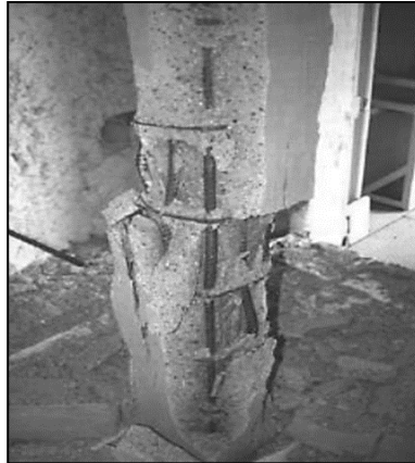
Figure 4: Example of explosive spalling occurred in high strength concrete column (Kodur et al., 2005).
